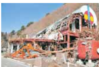
The underground aquarium was completely destroyed including its office facility on the ground.
