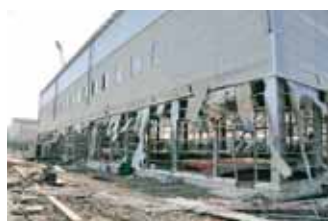
Shipbuilding factory also had serious damages.
